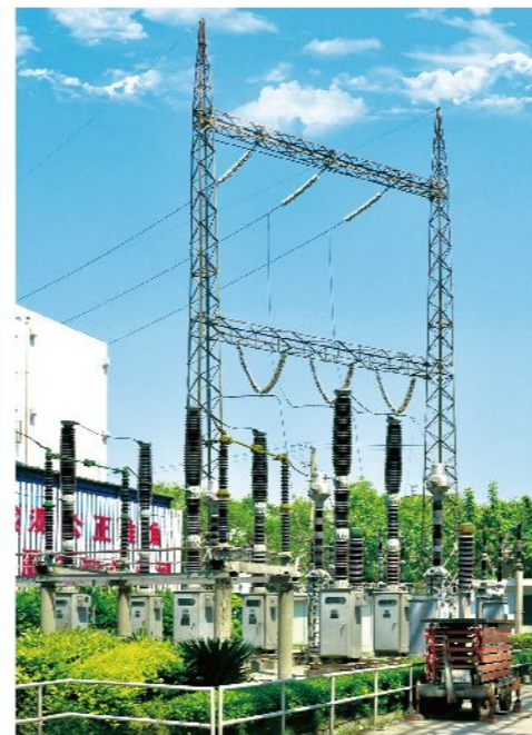
220kV 户外开关站 220kV Outdoor Switching Station
